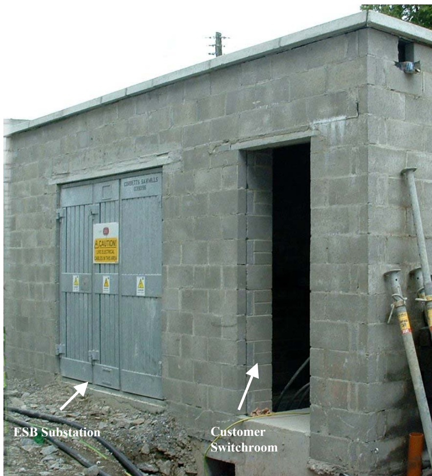
Fig. 1 Freestanding MV Substation
