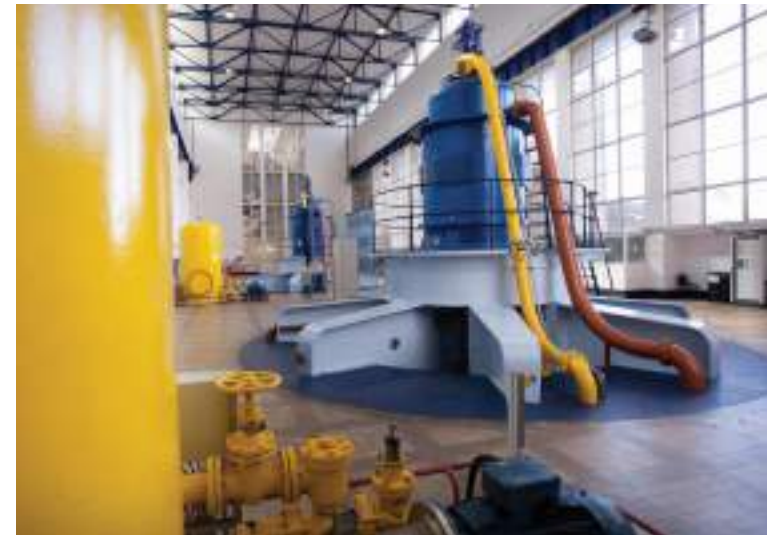
Generator Floor, Cathaleen's Fall Generating Station.
